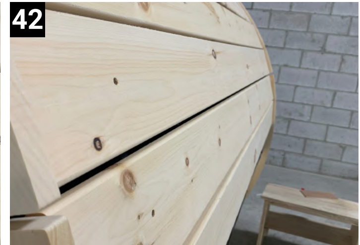
42 About 1/4" spacing between roof boards
