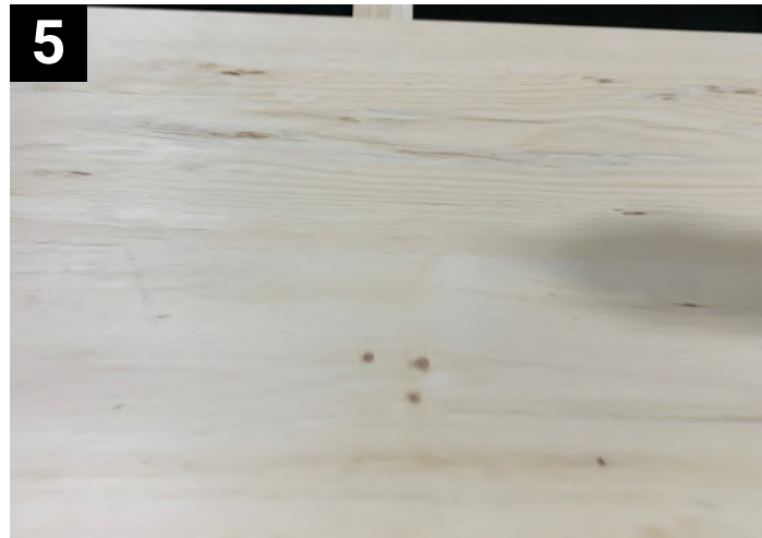
5 No screws in Center isle way.
