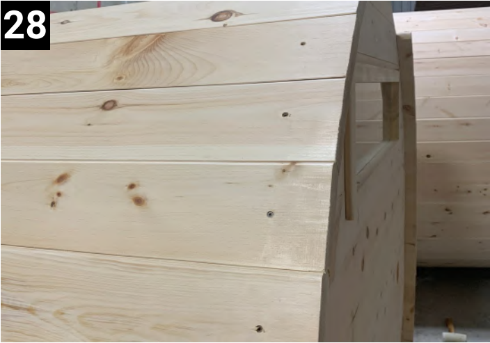
28 Put staves on and fasten on. Leave the last 8 staves unscrewed to allow putting in the top stave
