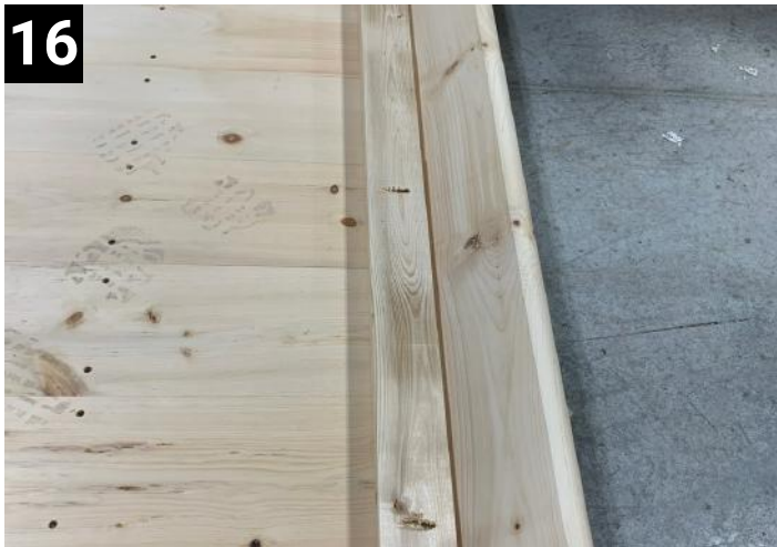
16 Put in long floor cleats and screw down into floor and into staves
