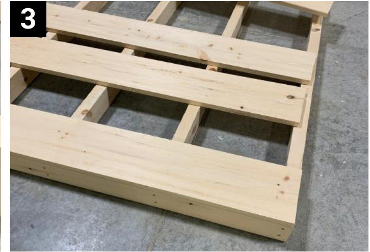
3 Lay floor boards on and start at one end and screw it down. Keep floor boards as tight together as possible
